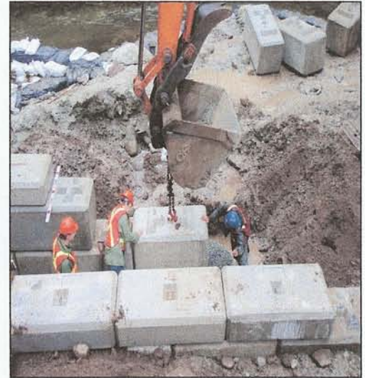
Engineers carefully place blocks that make up the sides of new fish trap.
