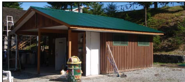
The Allco Fish Hatchery Incubation Room with a new roof. The old roof was leaking and in need of great repair to ensure damage was not done to the building interior.
